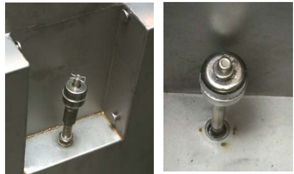
Figure 1: The float switches (above and right) should be cleaned periodically to eliminate starch buildup, which can impede the motion of the floats. Care must be taken, however, to ensure the shafts are not dislocated or the movement of the float hindered.
