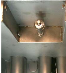
Upper float switch.
